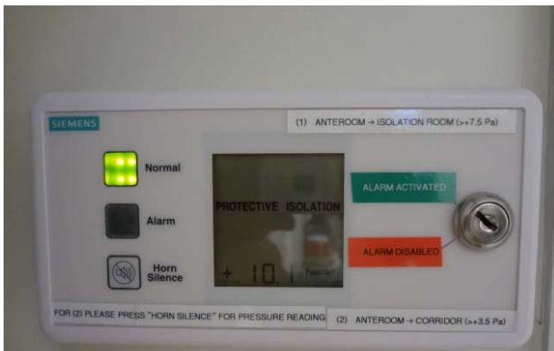
Isolation room monitoring panel
