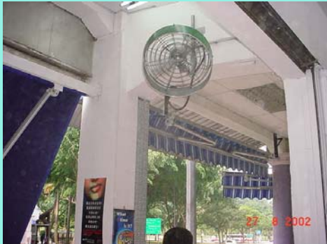
wall-mounted mist fans
